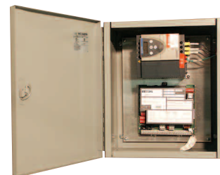
Electrical Control Box
